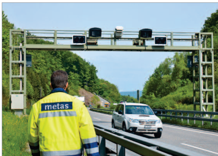
Figure 2 ASC gate on the A2 highway at the entrance to the Arisdorf tunnel
